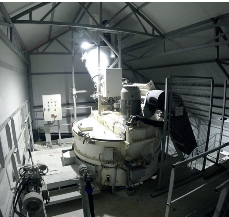
Mixer platform in a cladding
